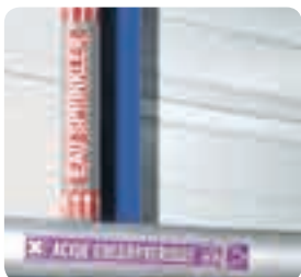
Identify pipelines on-site
